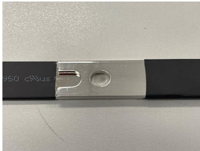
GOOD - No heatshrink tubing between conducting surface of busbars
