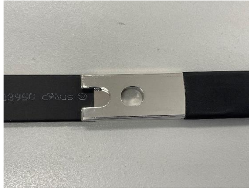
UNACCEPTABLE - Heatshrink tubing between conducting surfaces of busbars
