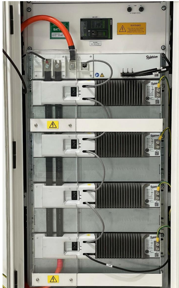
Battery D.C Isolator (MCCB1)
